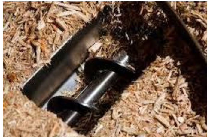
Wood chip boiler and wood chips feeding to boiler/ Comparison Of Wood Chip And Wood Pellet Installations
