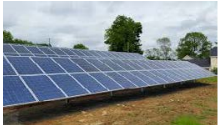
50kW Photovoltaic. Image from Solmatix Renewables
